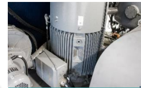
Predictive Maintenance of Drives (Edge Comp.) 2 5
